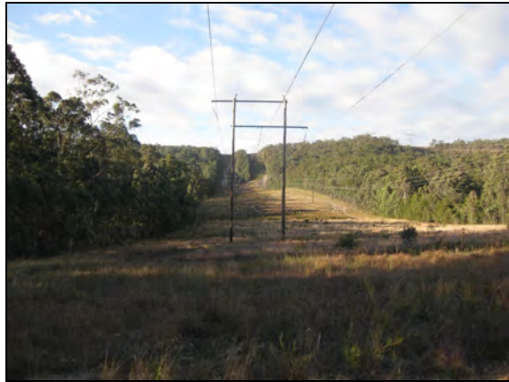
Ausgrid 132 kV Transmission Line Easement*
