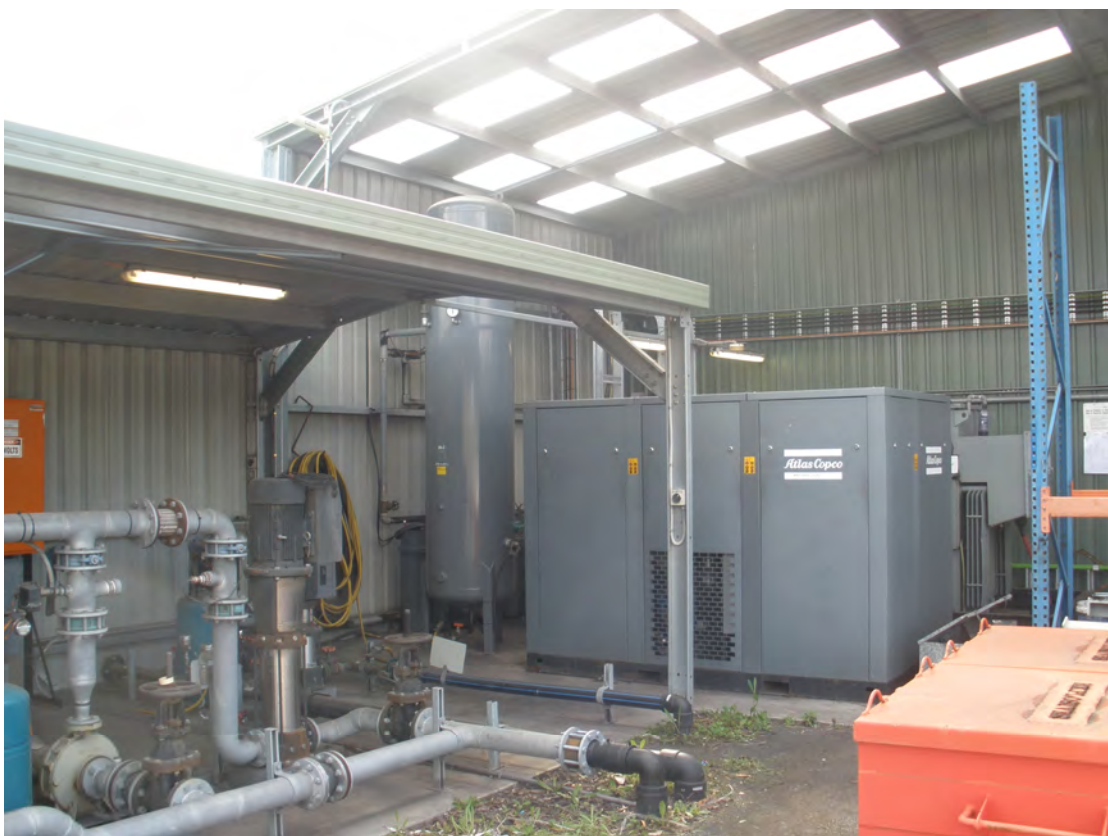
Plate 8 - Mine services area - pumps, air compressors and electrical equipment
