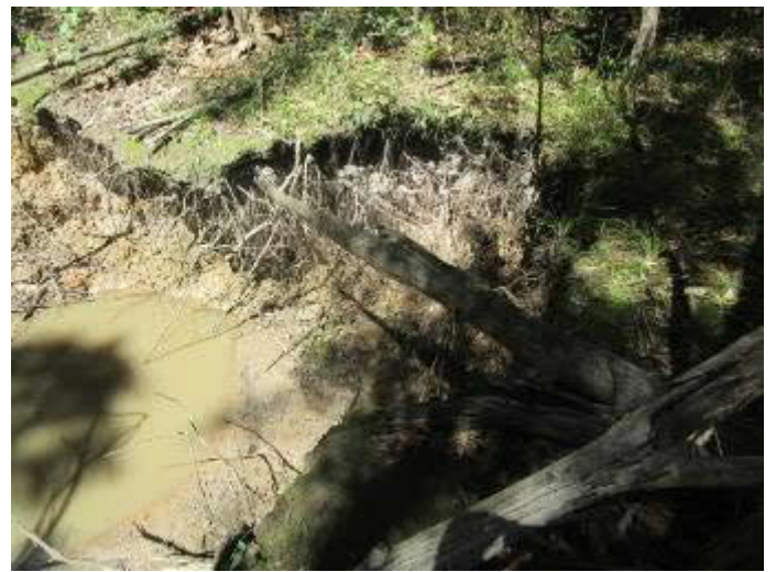
Plate 82 – Erosion Downslope of Sediment Dam E
