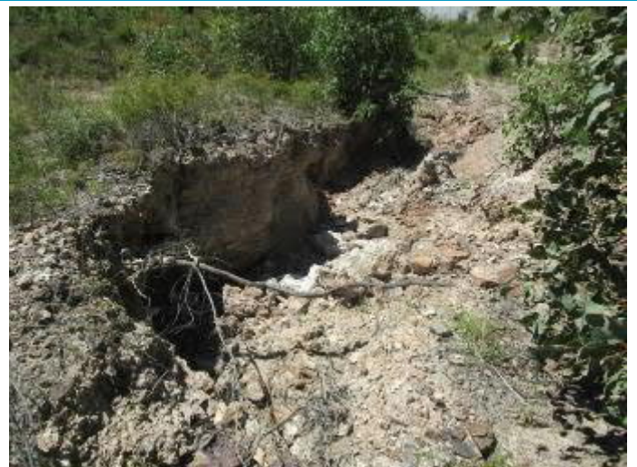
Plate 96 – Eroded Channel Upslope of Rumbles Dam
