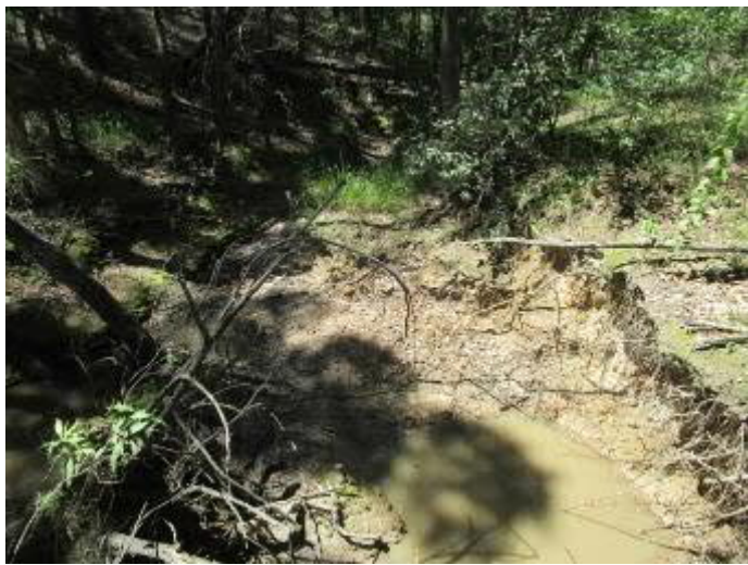
Plate 81 – Erosion Downslope of Sediment Dam E
