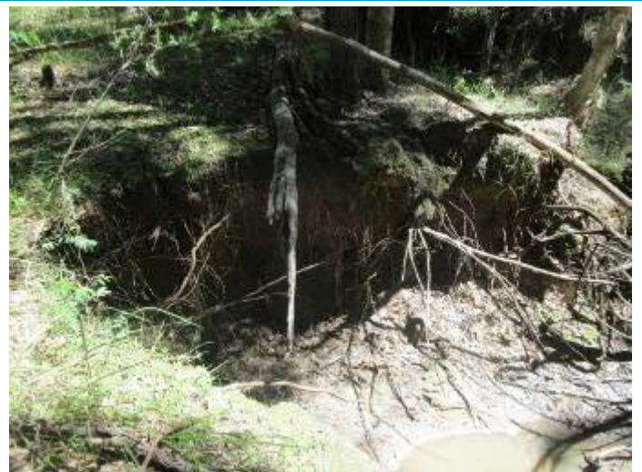
Plate 84 – Erosion Downslope of Sediment Dam E
