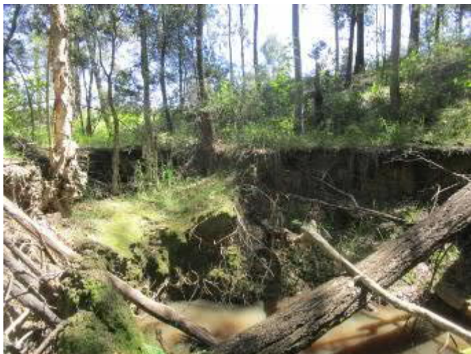
Plate 87 – Erosion Downslope of Sediment Dam E
