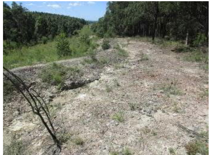
Plate 92 – Eroded Channel Upslope of Rumbles Dam
