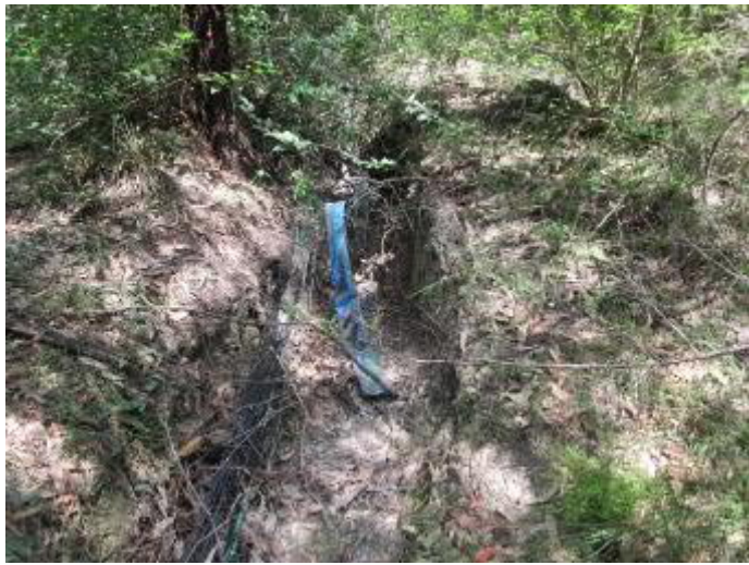
Plate 108 – Erosion Downslope of Rumbles Dam
