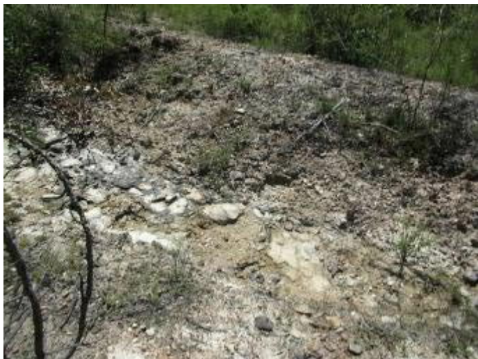
Plate 93 – Eroded Channel Upslope of Rumbles Dam
