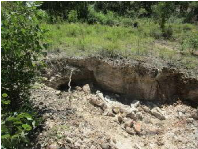
Plate 97 – Eroded Channel Upslope of Rumbles Dam
