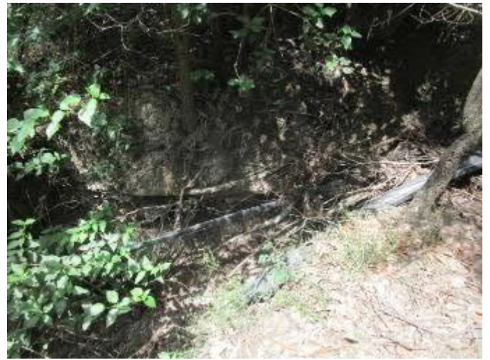
Plate 109 – Erosion Downslope of Rumbles Dam
