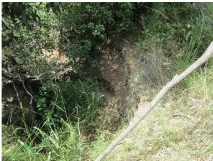
Plate 112 – Erosion Downslope of Rumbles Dam
