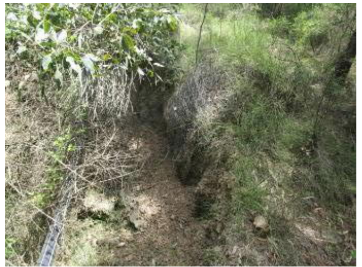
Plate 111 – Erosion Downslope of Rumbles Dam
