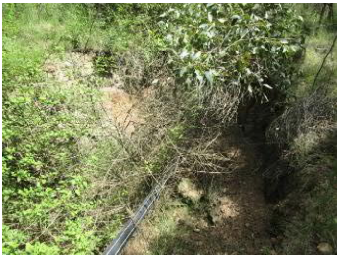
Plate 110 – Erosion Downslope of Rumbles Dam
