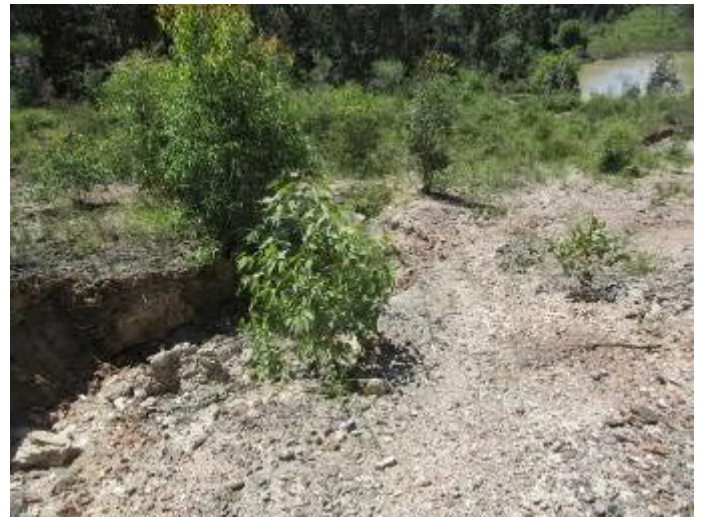
Plate 98 – Eroded Channel Upslope of Rumbles Dam
