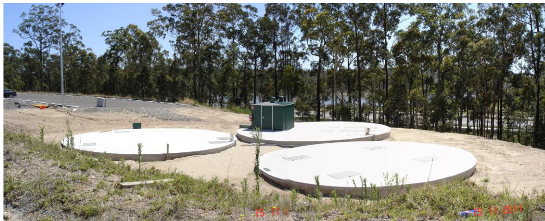
Plate 3: Tertiary Treatment System installed in 2011 – rehabilitation of the area around the in-ground tanks is planned for 1Q 2012.
