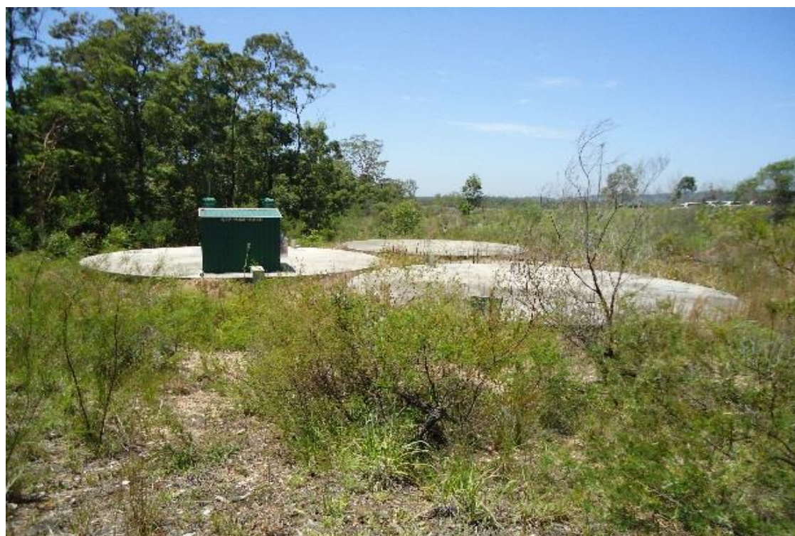
Plate 18 Well managed wastewater treatment area
