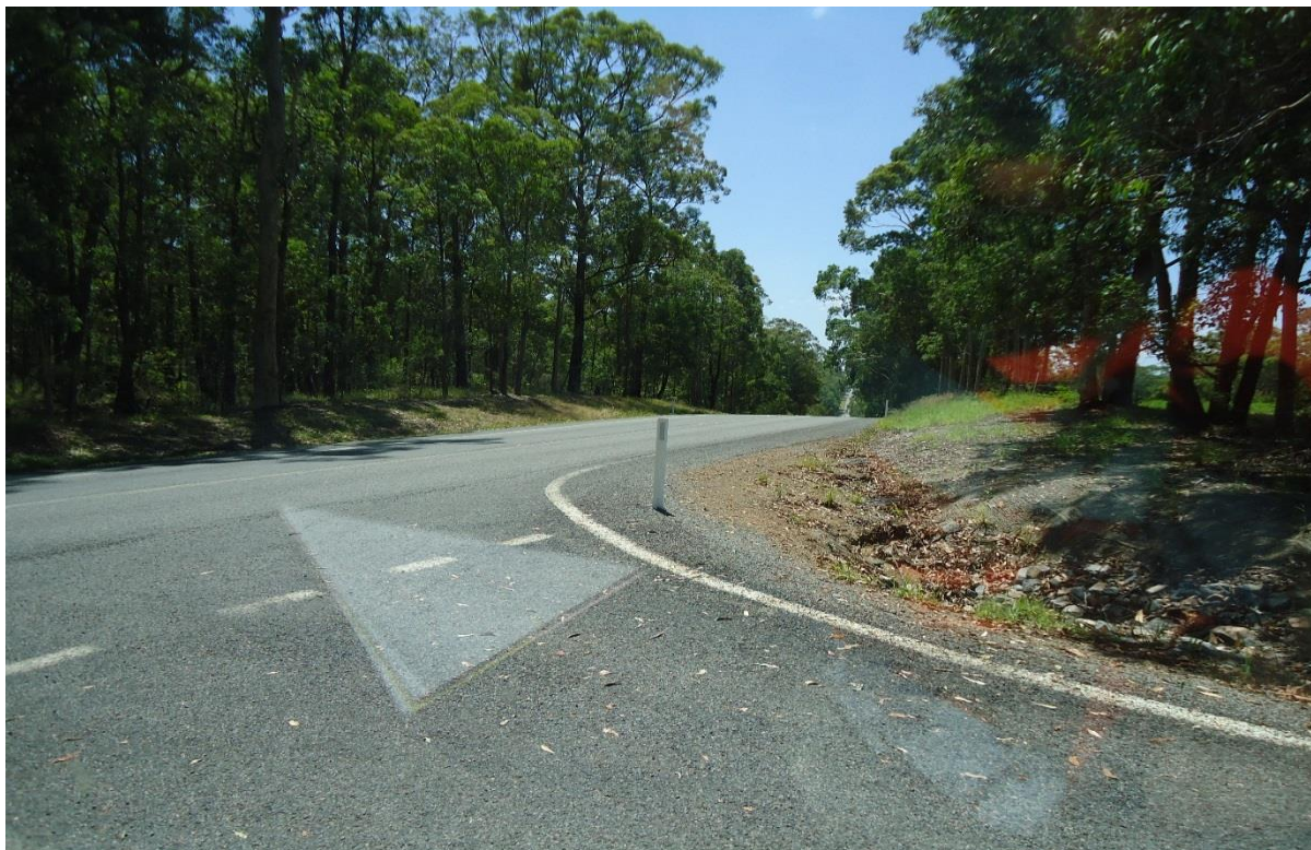
Plate 9 Meredith Road where remediation conducted after subsidence
