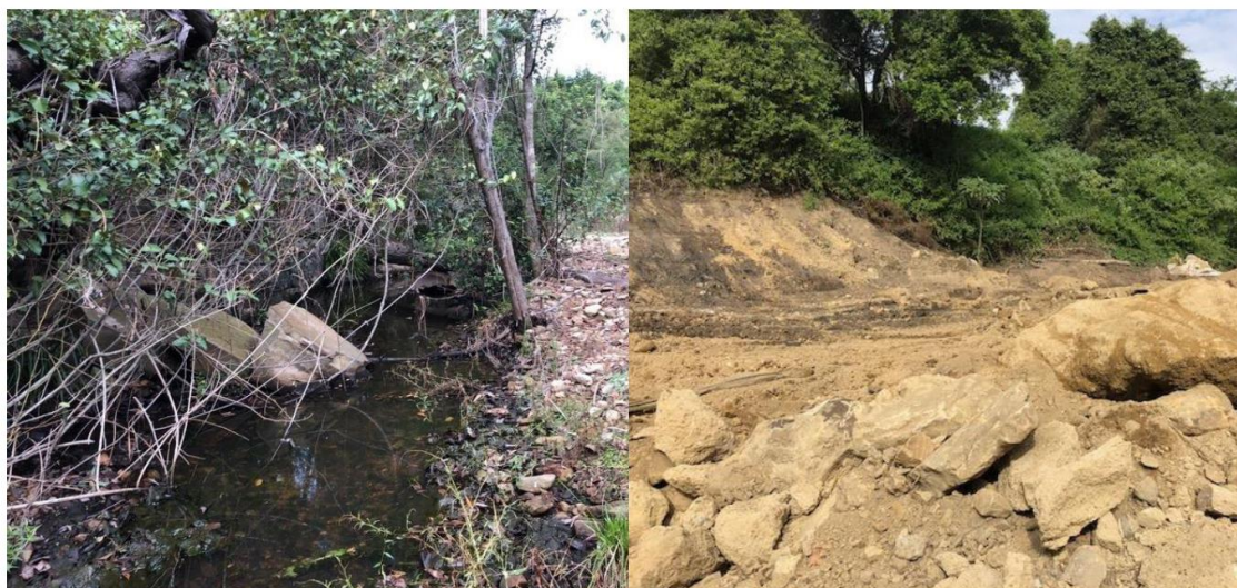
Plate 2. Blue Gum Creek at Stockrington Road. Left: sampling site. Right: Bridge repair work upstream.
