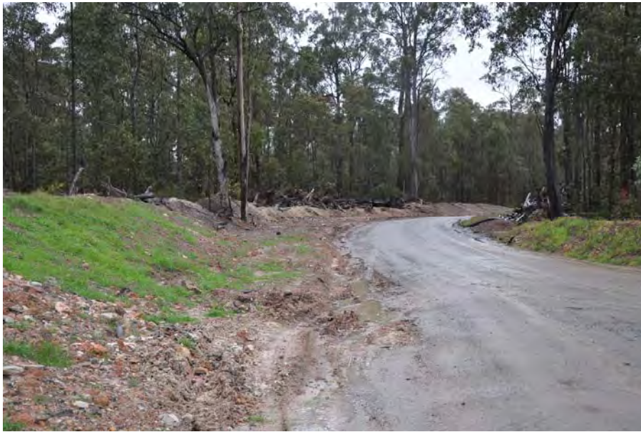
Plate 1 View east across the widened substation access road (Date of Photography 10 August 2010)
