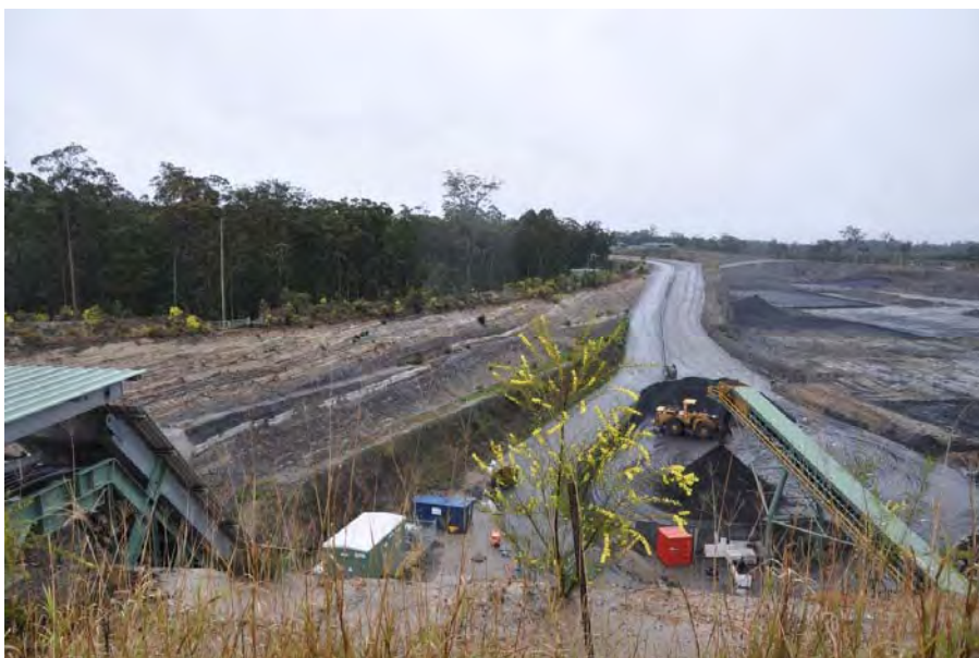
Plate 3 View north over portal and coal handling area (Date of Photography 10 August 2010)
