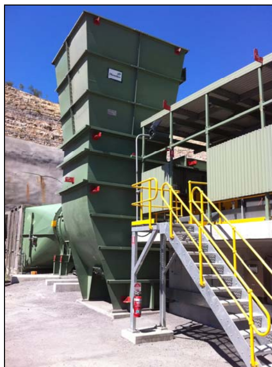
Plate 3 Existing Ventilation Fan in Abel Box Cut
